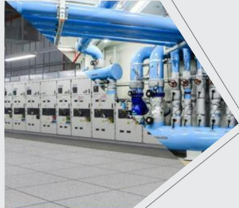
Electrical & Mechanical Contracting Operation & Maintenance
